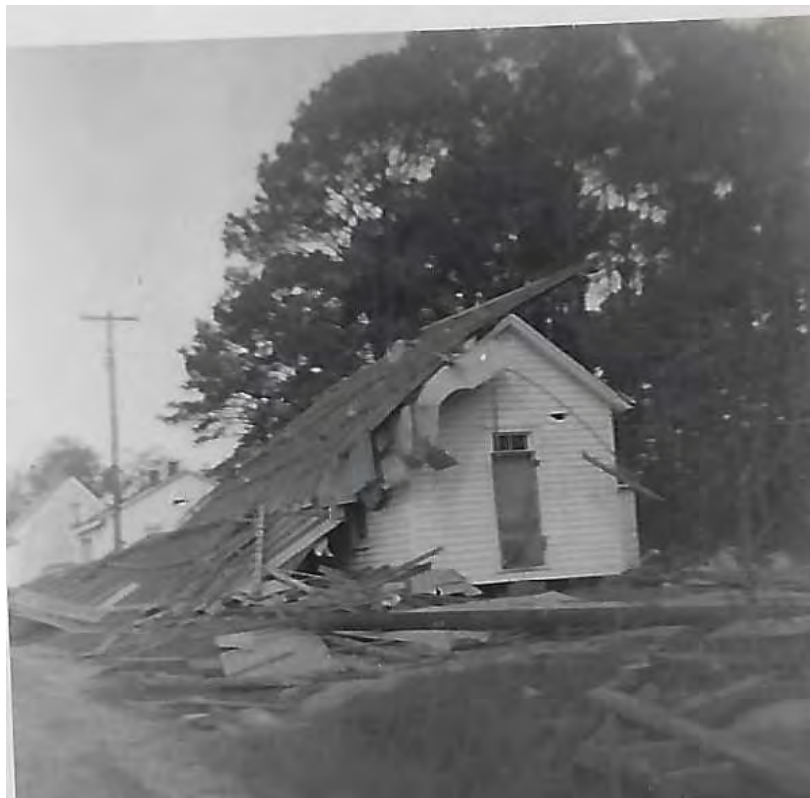
Figure 6: Wind Damage from the Hurricane of 1933. Photo Credit-Unknown
