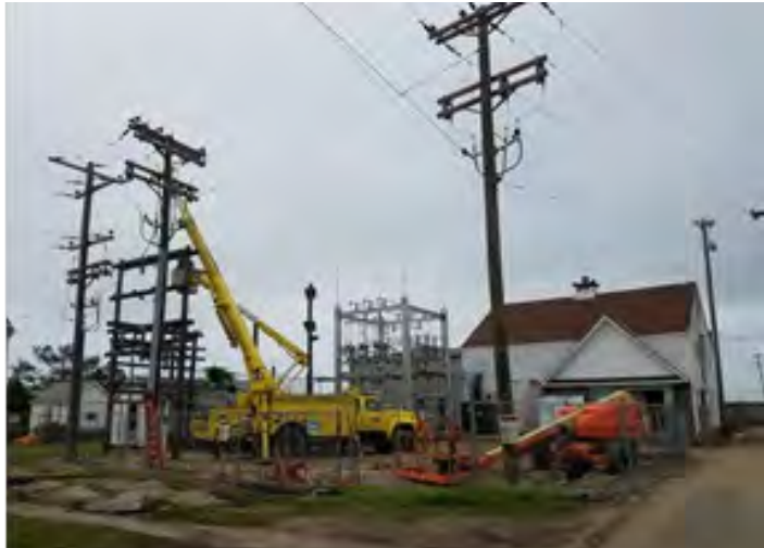
Figure 7: Electric substation. Photo by Shannon Alexander
