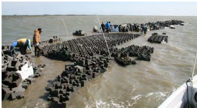
Figure 11: Oyster Reef under Construction Photo Credit: © Bowdoin Lusk/ The Nature Conservancy. Used with permission.
